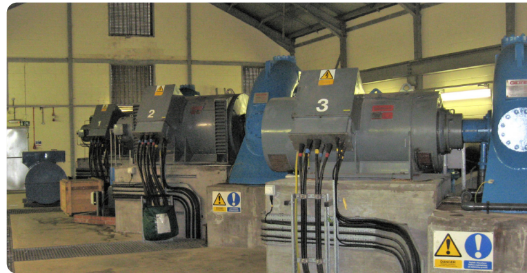
Electricity at Llyn Brianne hydro scheme is generated by three turbines.
