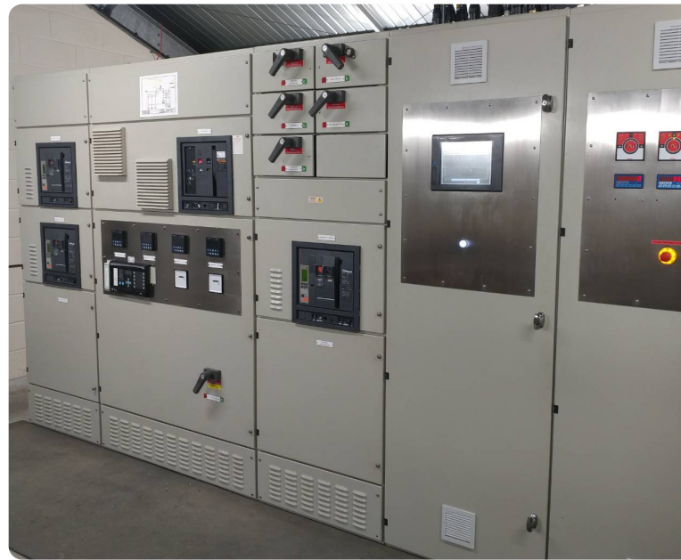
The adaptations to the existing control panel were constructed offsite, reducing the time required for installation. Using this method reduced the necessary downtime at the plant by between a month and six weeks.
