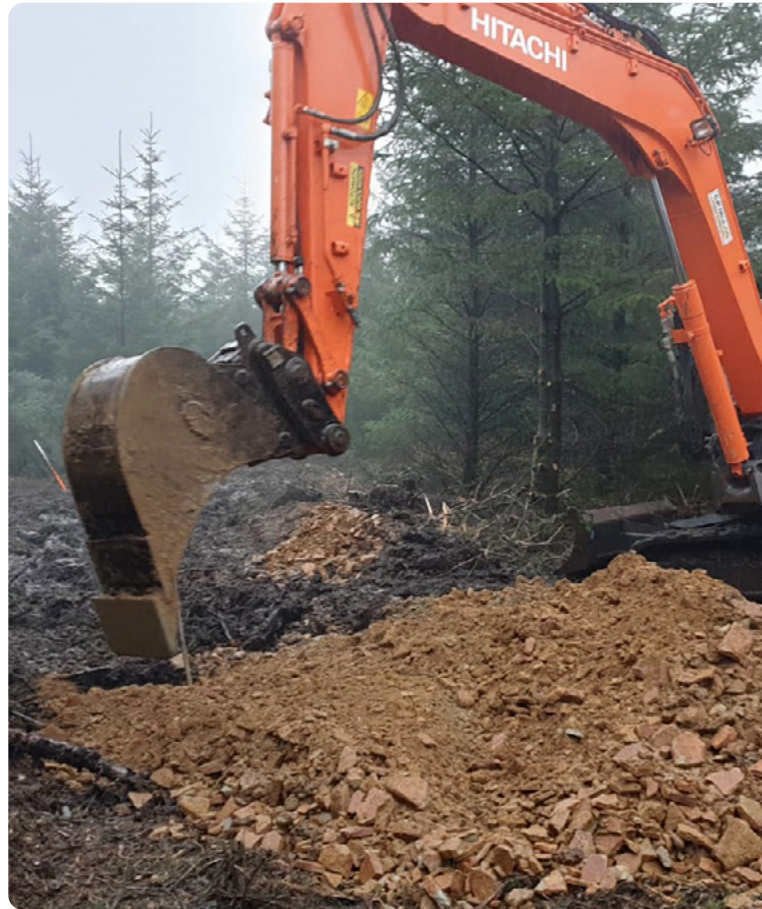
Groundwork preparation for anchor installation, set within a clear-fell area of forestry land.
