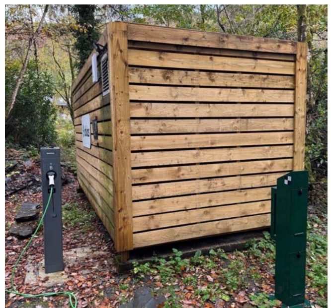
Dual EV and E-bike pedestal chargers connected to the containerised battery in the tricky wooded location.
